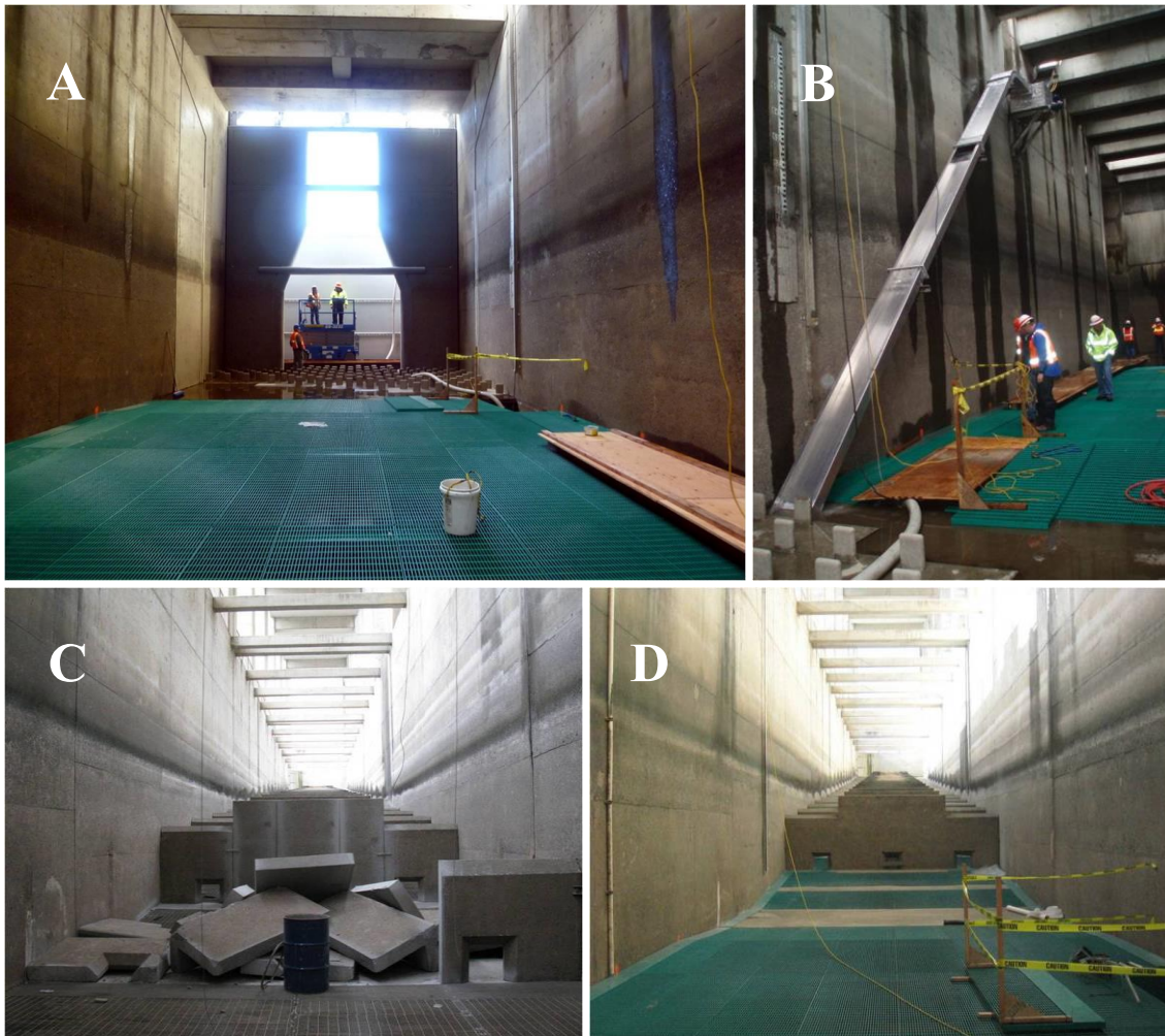
Figure 15. Modifications to the John Day Dam north fishway entrance area; camera is facing upstream in all photos except A. From left to right, clockwise: A) downstream variable-width entrance weir, bollard field, and closed entrance slot (new concrete on left wall); B) lamprey passage structure (with bollard field in foreground); C) removal of concrete weirs; and D) completed fishway with concrete weirs removed.
