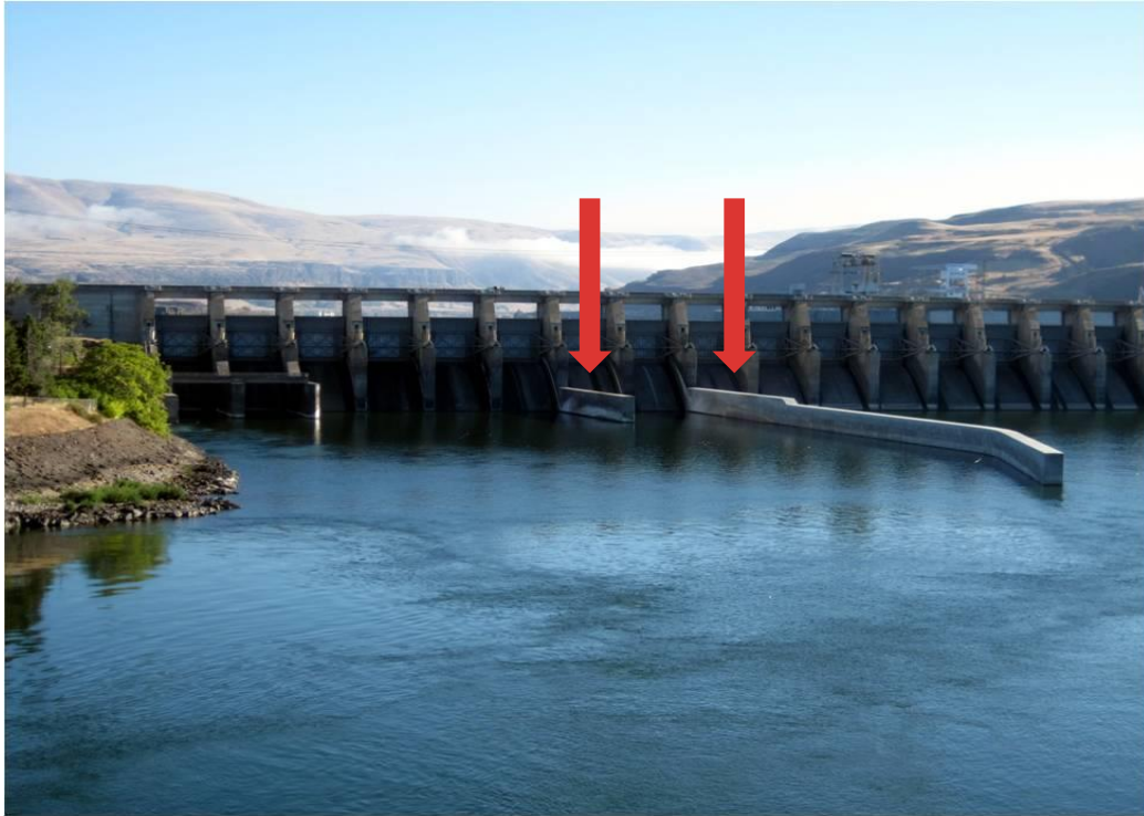
Figure 1. Photograph of spill walls at bays 6-7 (left arrow) and 8-9 (right arrow) at The Dalles Dam in 2010.
