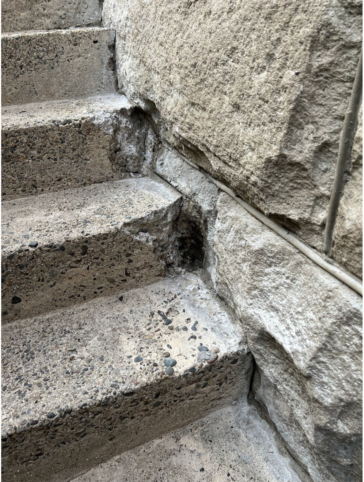
Figure 2 Deterioration at stairs
