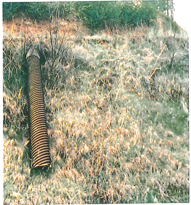
In unstable soils, direct outflow from a culvert away from potential damage.
