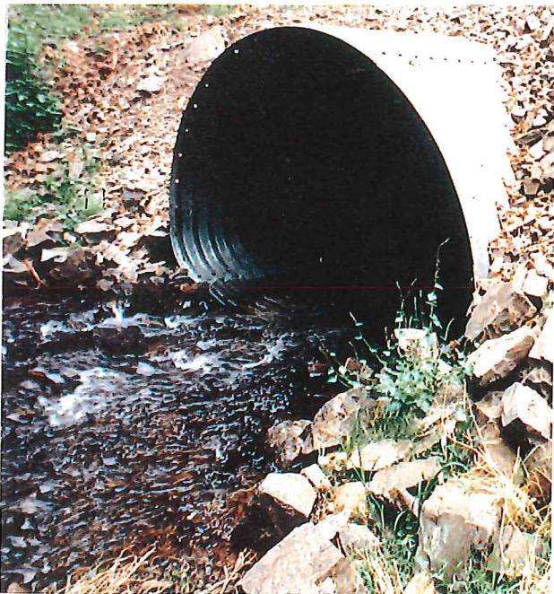
A culvert must be properly laid in the stream bed. Obtain all permits before beginning.
